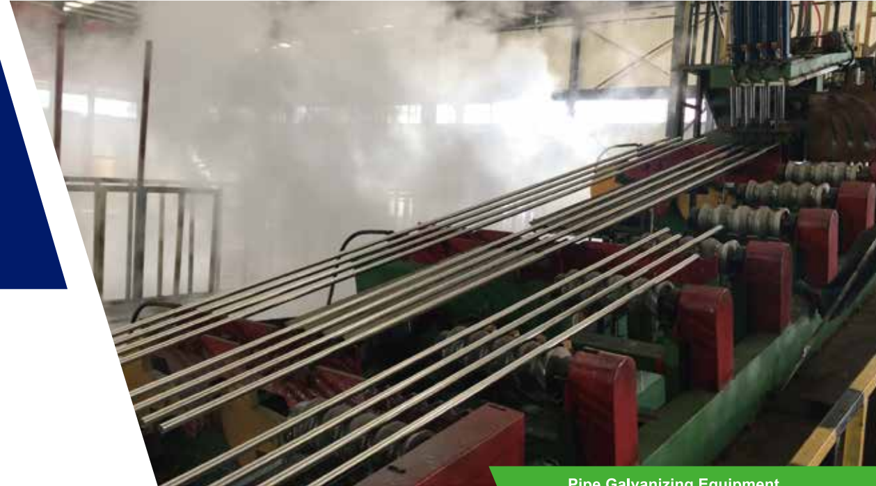
Pipe Galvanizing Equipment
